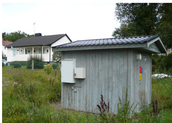
Odour removal for pump stations close to other buildings
